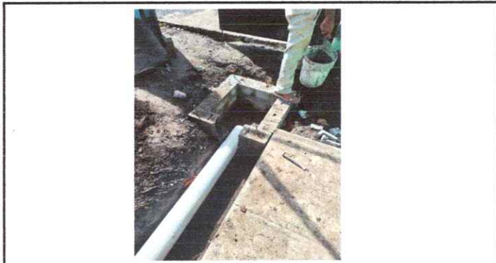
Foto 9: Drenaje colapsado, Region 19.18 (Instalacion de tuberia principal PVC)
