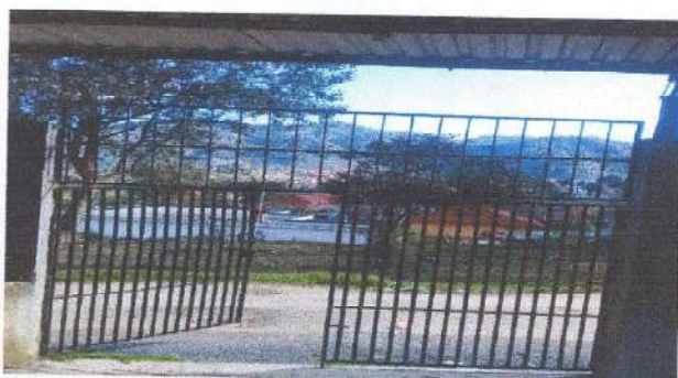
Foto 10: Porton principal inestable
