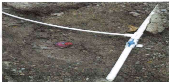
TUBERIA PRINCIPAL DE AGUA POTABLE
